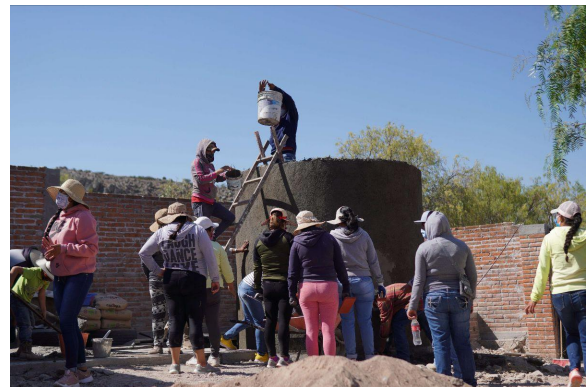
Photo: A group of community members from La Norita del Refugio building a Rainwater Harvesting System.
