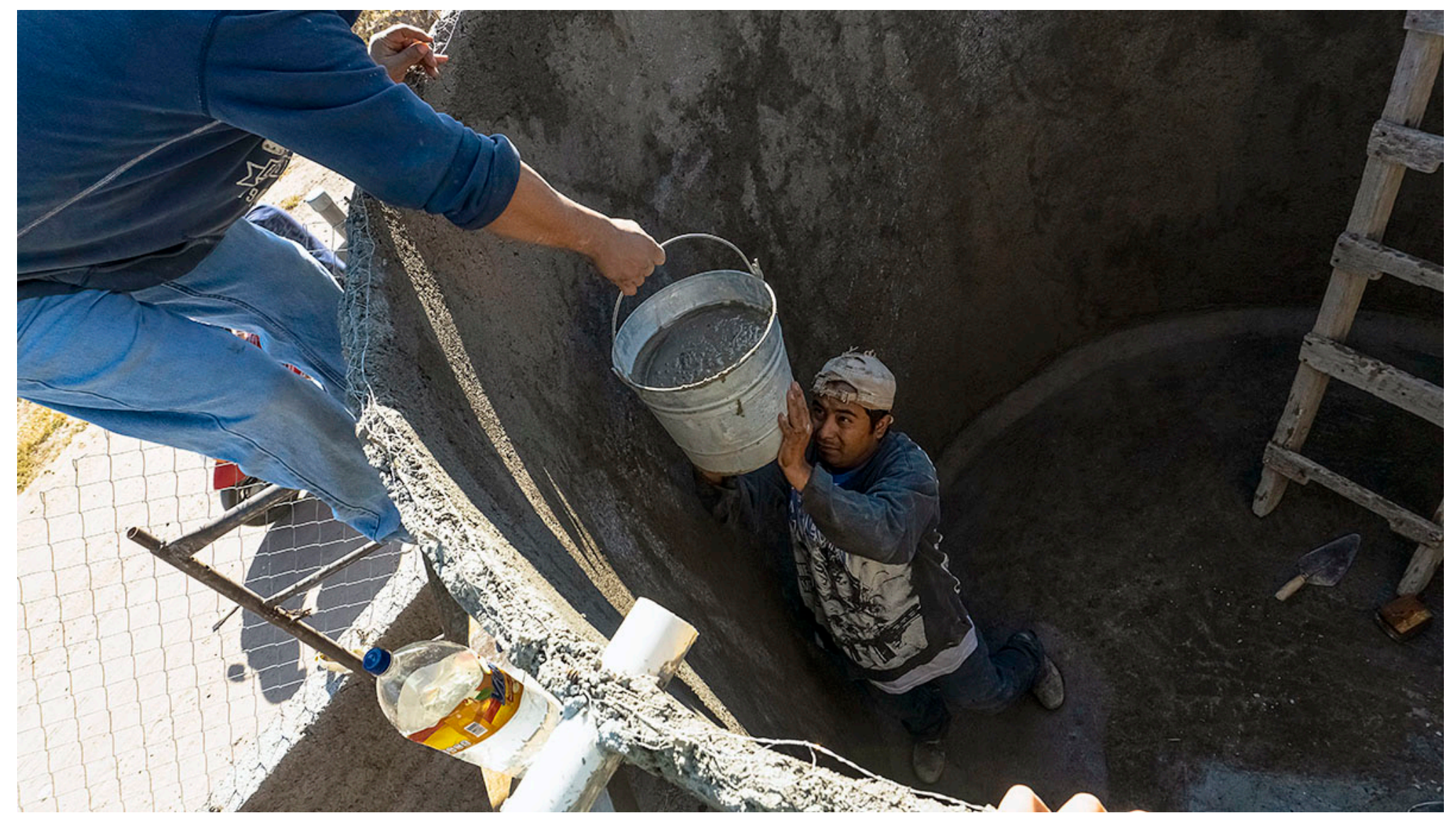
Photo: Two community members working on the construction of a rainwater harvesting system.
